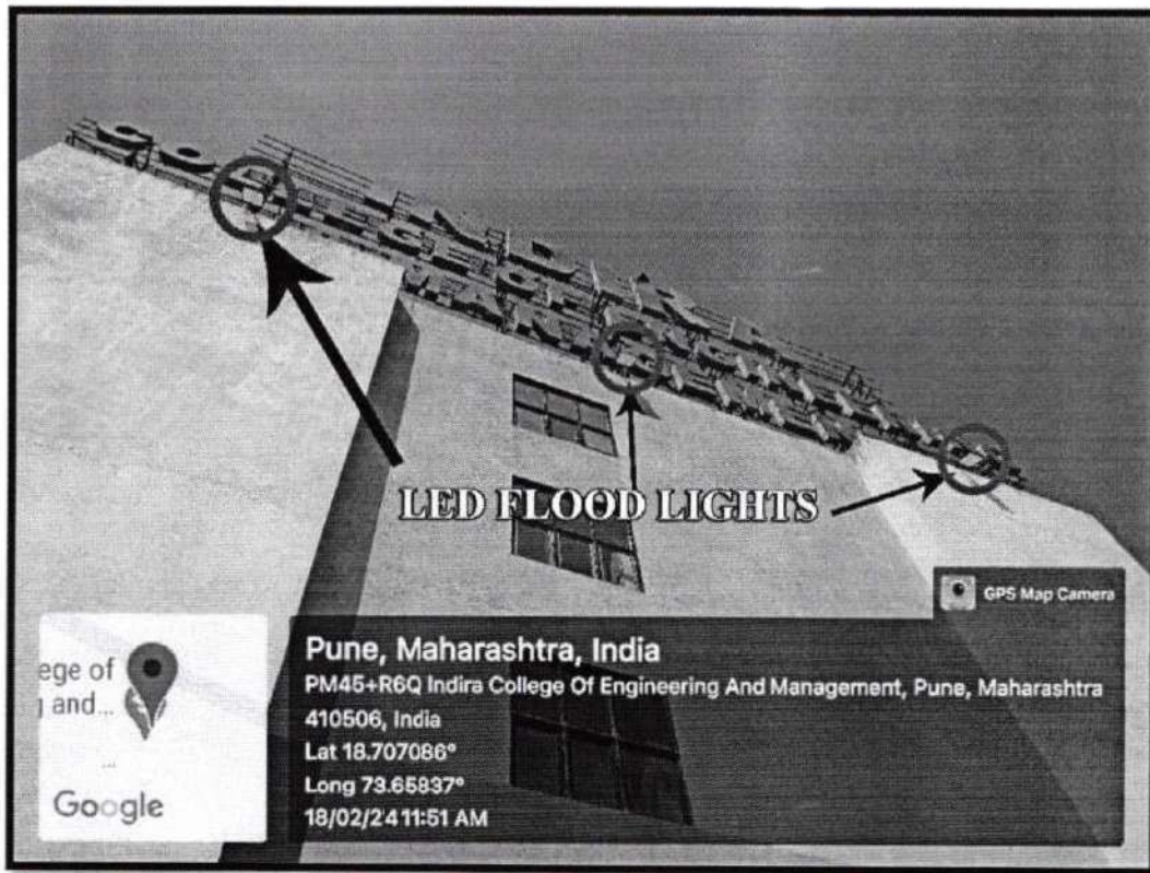
Photo 03: LED Flood Lights at B Building
