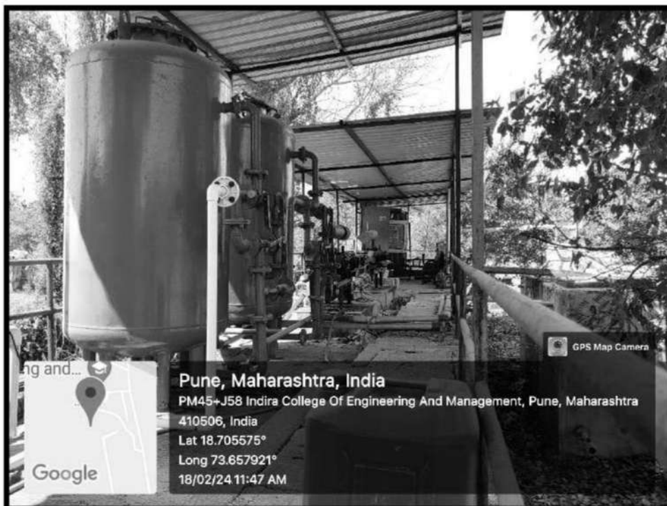
Photo 04: Pressure Sand Filter and other units of Waste Water Treatment Plant
